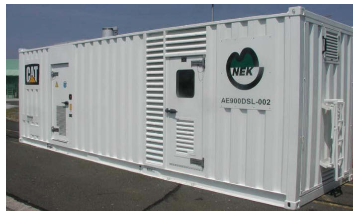
Portable external diesel generators
