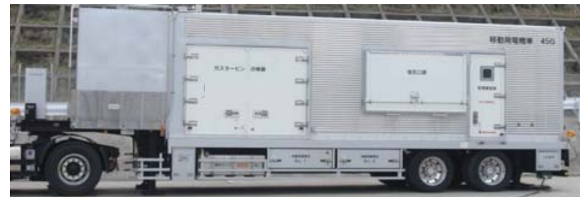
Alternative onsite AC power (Power Vehicle)
