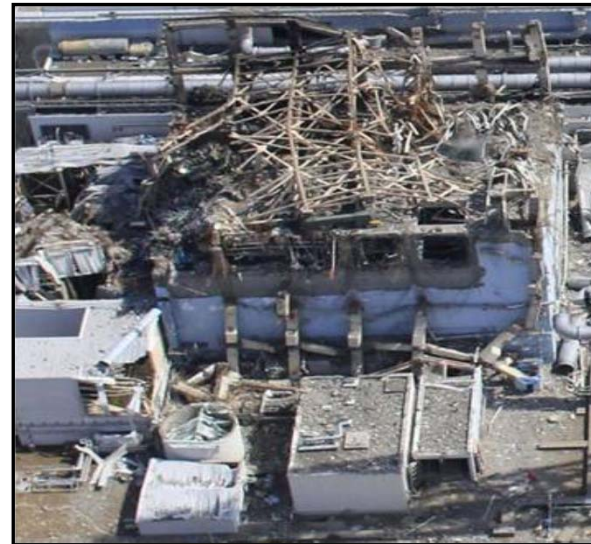
The severely damaged RB of U3 due to the hydrogen explosion (Source: TEPCO)
